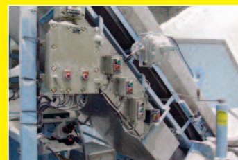
Sugar silo conveyor
