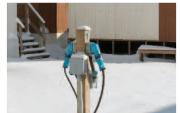
External power supply for water treatment
