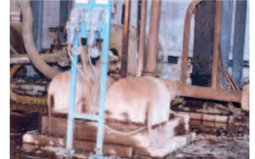
Pumps in wet atmosphere
